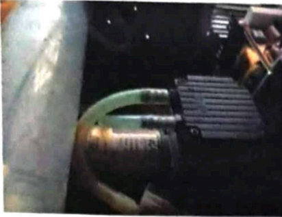
24V PUMP & TUBINGS
